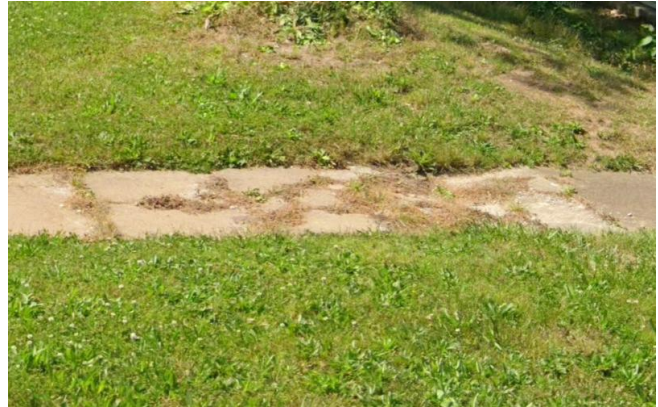
Poor Surface Condition
