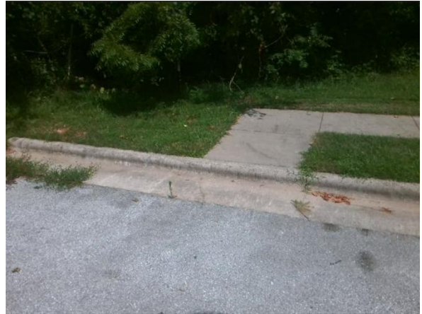
Missing Curb Ramp
