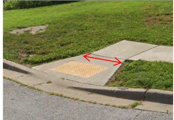
Curb Ramp Cross Slope
