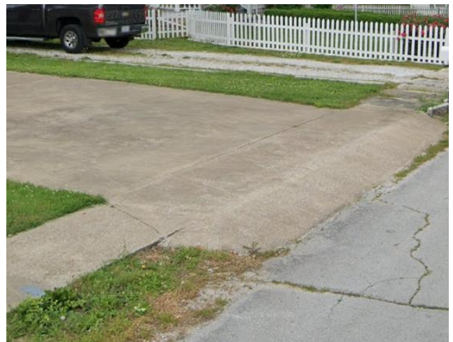
Sidewalk built through a driveway
